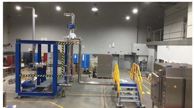
Frame with Turbines, Elec Panel, Recirc Pump, Connecting Pipework in place
