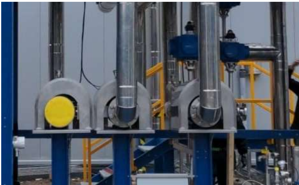
Figure 5. Side view of the demonstrator during assembly, showing the 3 Deprag turbine generator sets.
