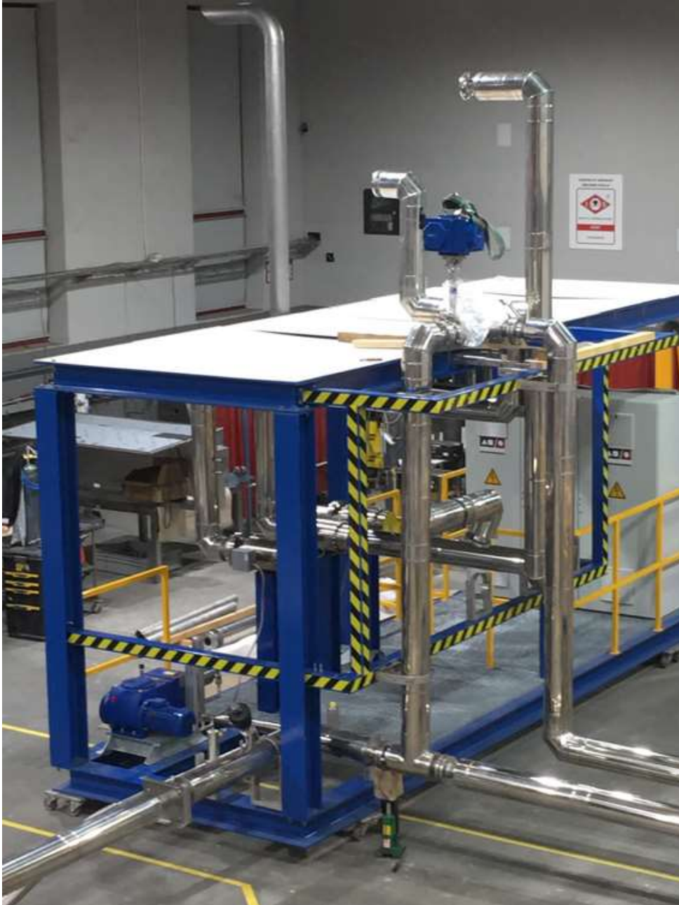
Figure 11. Demonstrator skid without the heat exchanger block.
