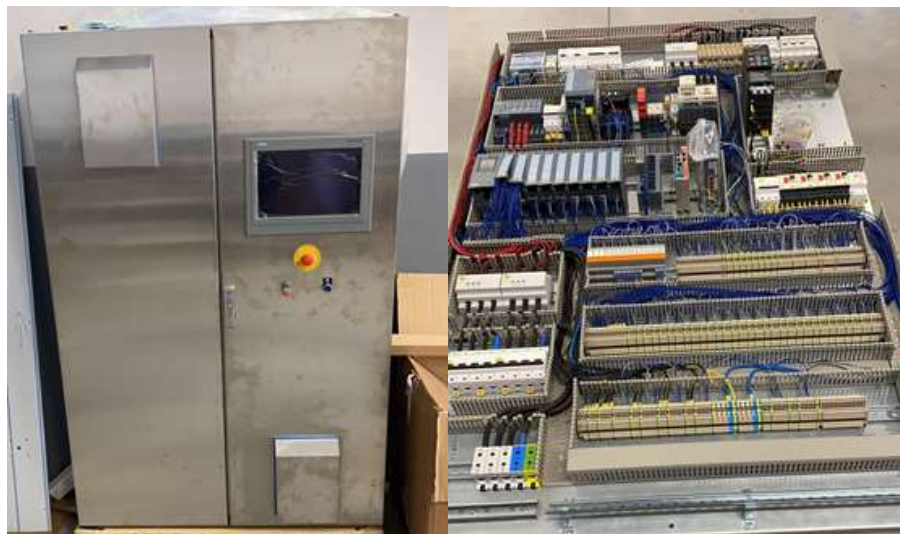
Figure 9. Electrical cabinet (left) and internal circuitry (right)
