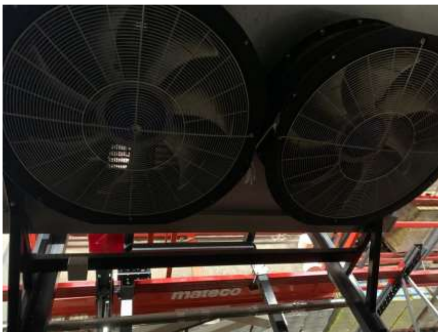
Figure 7. Heat exchangers mounted inside the warehouse.
