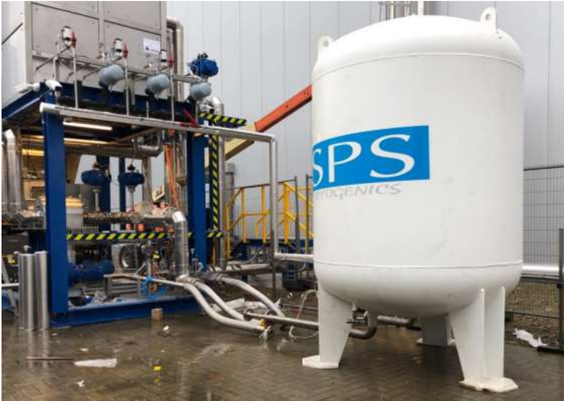
Figure 13. Side view of the demonstrator skid, with thermal store now delivered and ready for connection.
